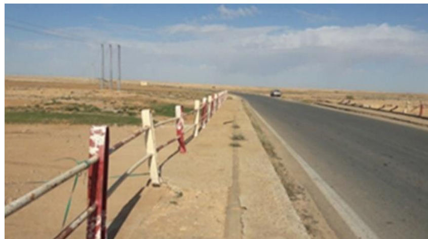
Figure 15 - Visual damage to bridge equipment. Source: Authors (2023).
