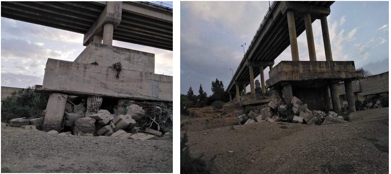
Figure 2 - shows the condition of the foundations of Baghlia Bridge.
